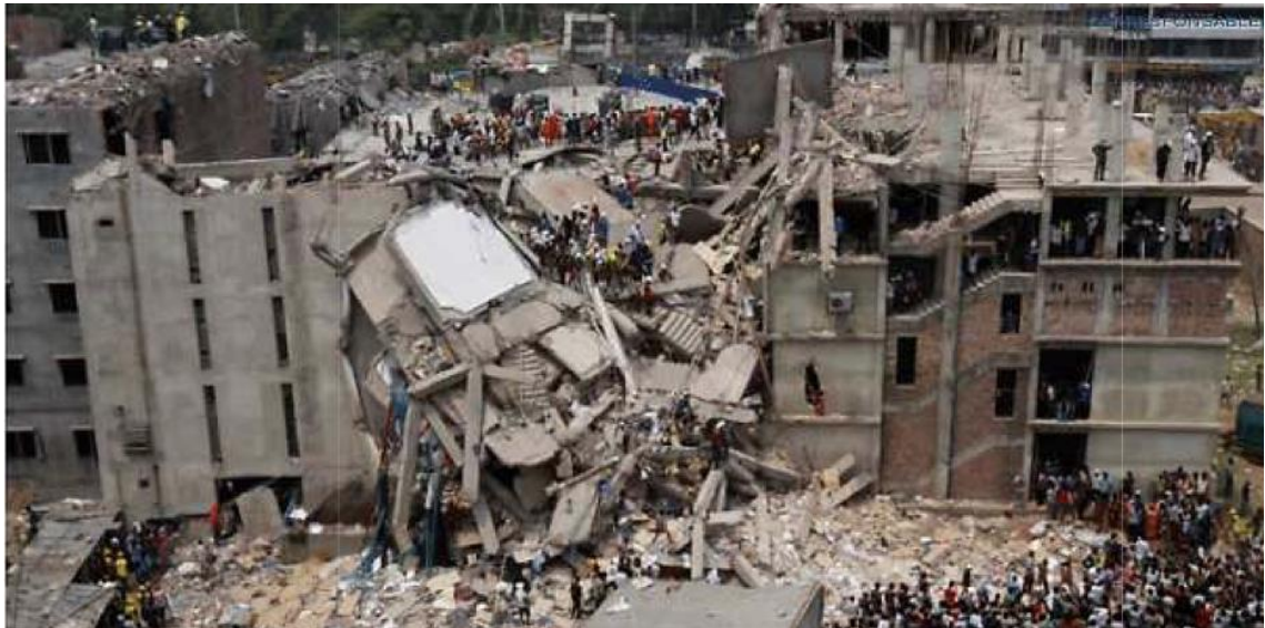
Figure 4: Bangladesh building collapse
